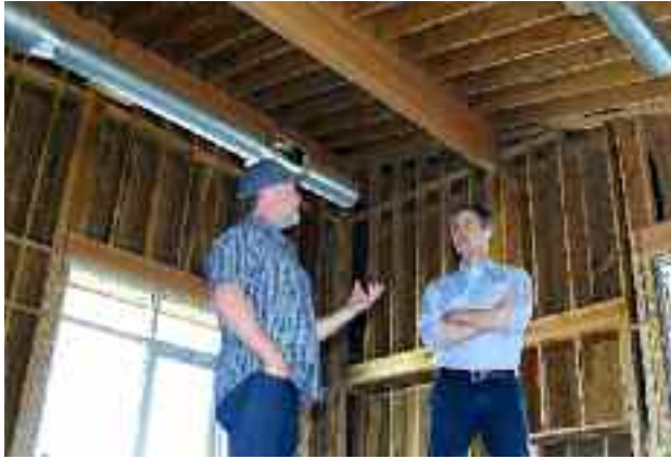
Senatorial candidate Beto O'Rourke (at right) is shown progress on the construction of a new restaurant on the grounds of Bonton Farms by Executive Director Daron Babcock (left). The eatery will feature food raised locally with the South Dallas farm. Babcock pledges the culinary product will be first-rate, hopefully bringing more awareness and popularity for the urban agricultural enterprise. (Photo: David Wilfong / NDG)
